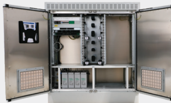
Cabinet with Batteries
