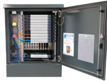
Fibre Distribution Terminal Cabinet iBER-835 G2 1x15U
