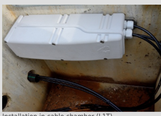
Installation in cable chamber (LIT)
